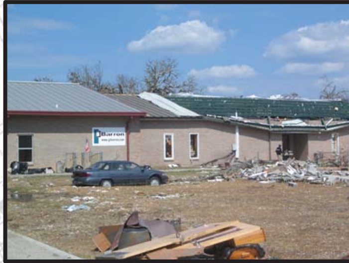
Damaged Classroom in Bay St. Louis next to Addition Barter & Associates Designed
