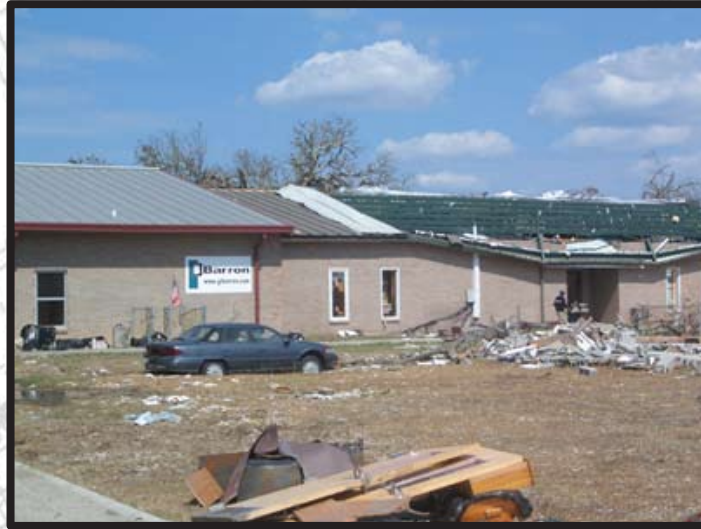
Damaged Classroom in Bay St. Louis next to Addition Barter & Associates Designed
