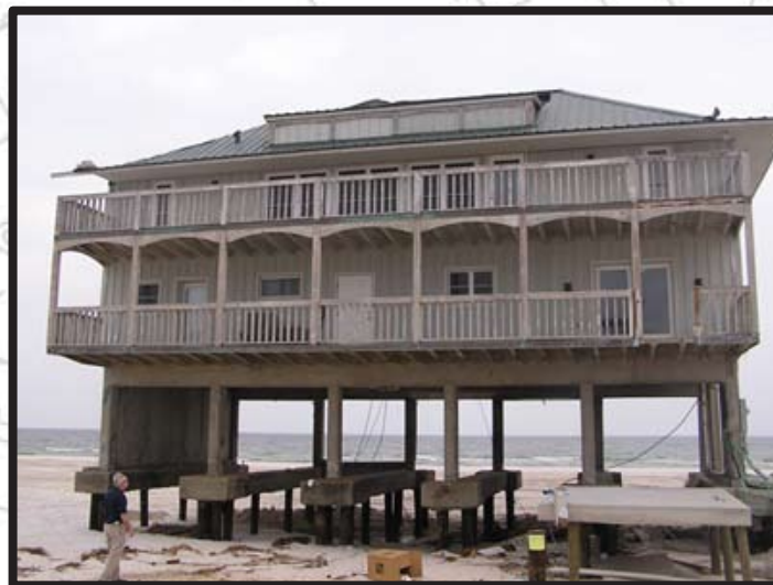
Residence Undermined by Storm Surge
