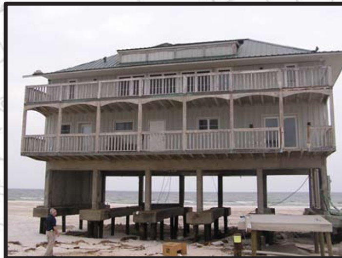
Residence Undermined by Storm Surge
